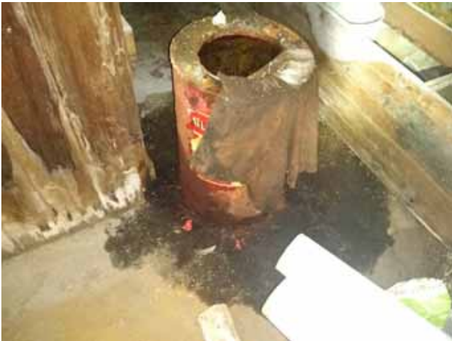
Photo 23: Oil staining around drum in basement (Parcel 2).
