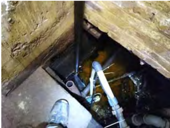
Photo 11: Apparent oil-impacted sump near central elevator (Parcel 1).
