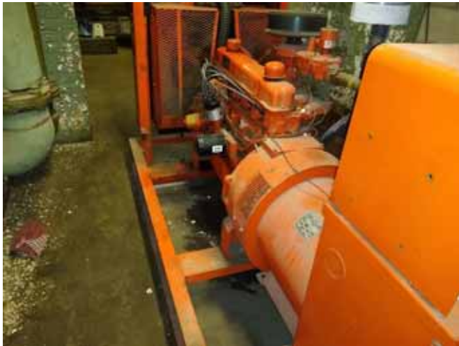
Photo 19: Oil staining on floor near compressor in basement (Parcel 2).
