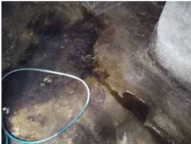
Photo 15: Floor drain with staining in basement (Parcel 1).
