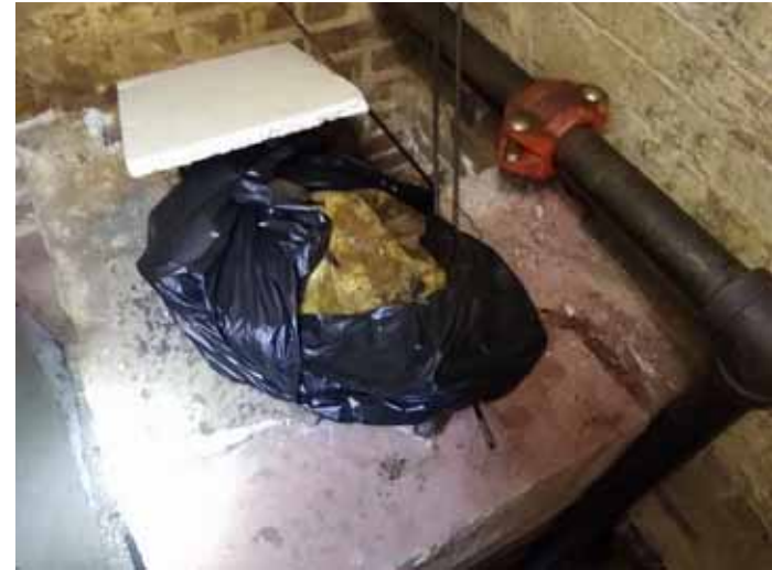
Photo 14: Oil-soaked pads adjacent to central elevator (Parcel 1).
