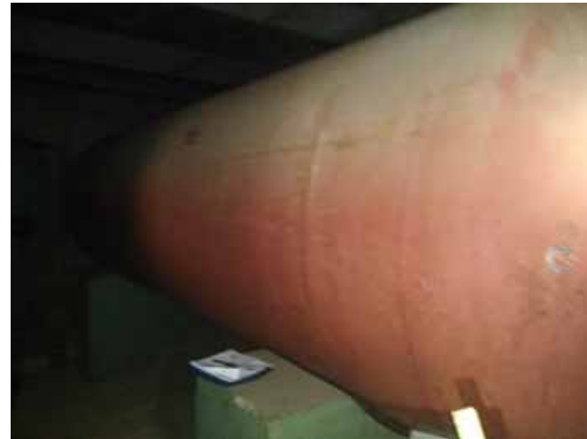
Photo 20: Approximately 5,000-gallon AST in basement (Parcel 2).
