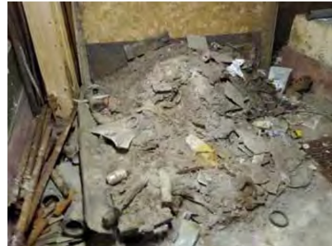
Photo 12: Debris pile in basement (Parcel 1).
