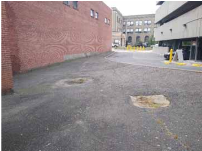
Photo 3: North wall of the Denholm building (Parcel 2), looking west. Worcester Plaza parking garage on right.
