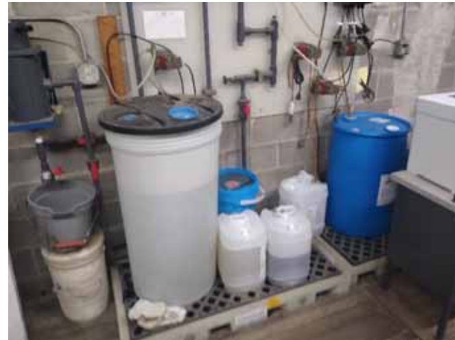
Photo 24: Heating system water treatment area in basement (Parcel 2).
