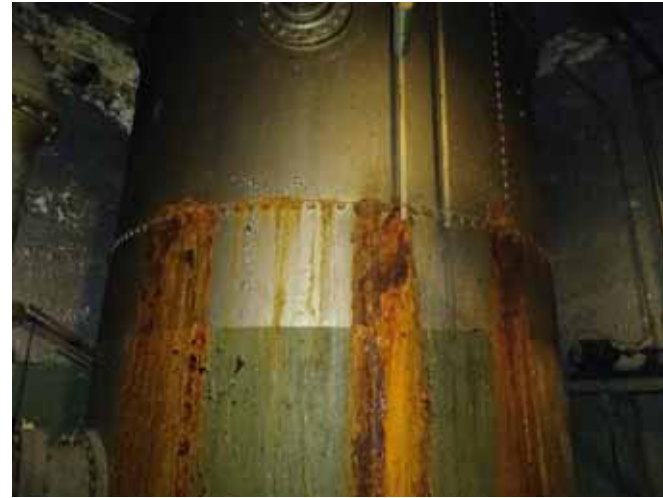
Photo 18: Reinforced upright steel tank in basement (Parcel 2).
